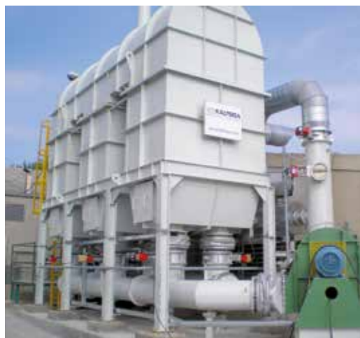
➤ Recuperative thermal oxidation
